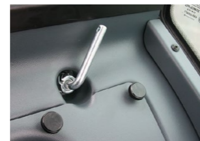
Battery master switch
